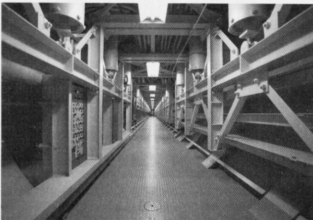
The cableway between the silo and the LCC
